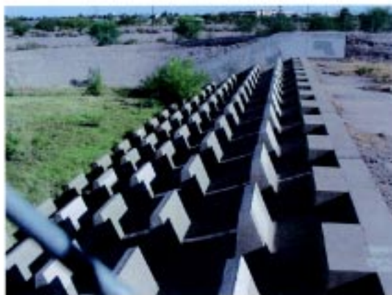
#28: Energy dissipators @ West Branch and Santa Cruz intersection (view to S)
