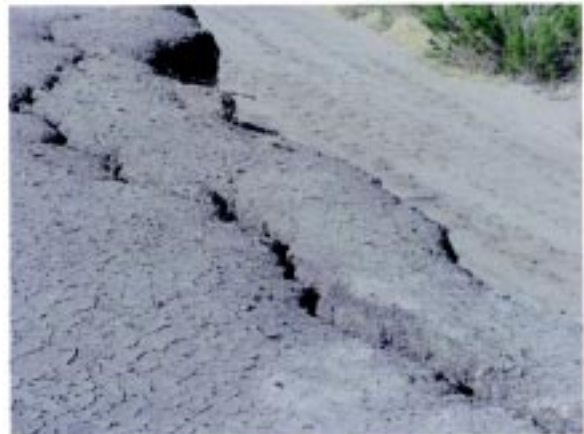
#19: Tension Cracks in W. bank, just S. of Valencia
