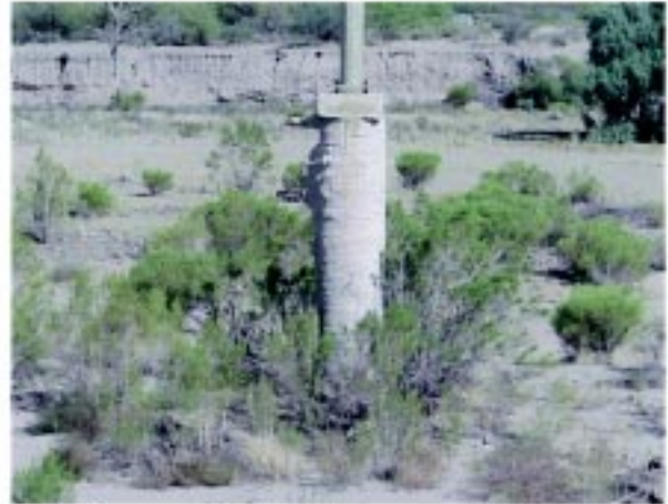
#14: Same pole foundation as previous showing bed degradation
